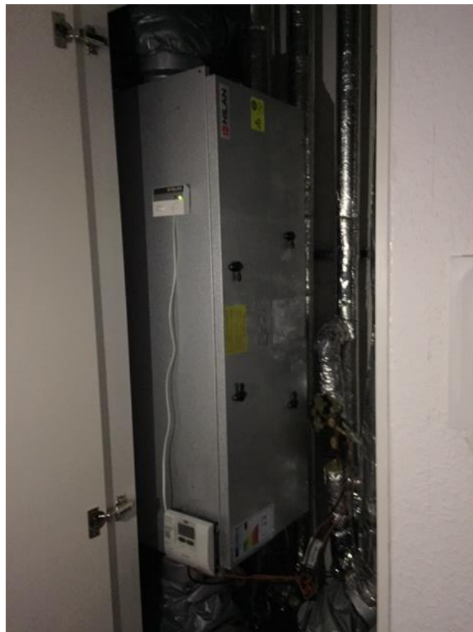
Figure 18: Ventilation heat recovery device in Building at RDS DK2
