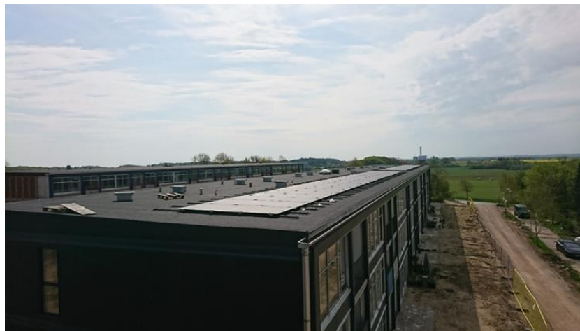
Figure 20: PVT system (RDP DK-PVT) installed on Trigeparken (RDS DK2)
