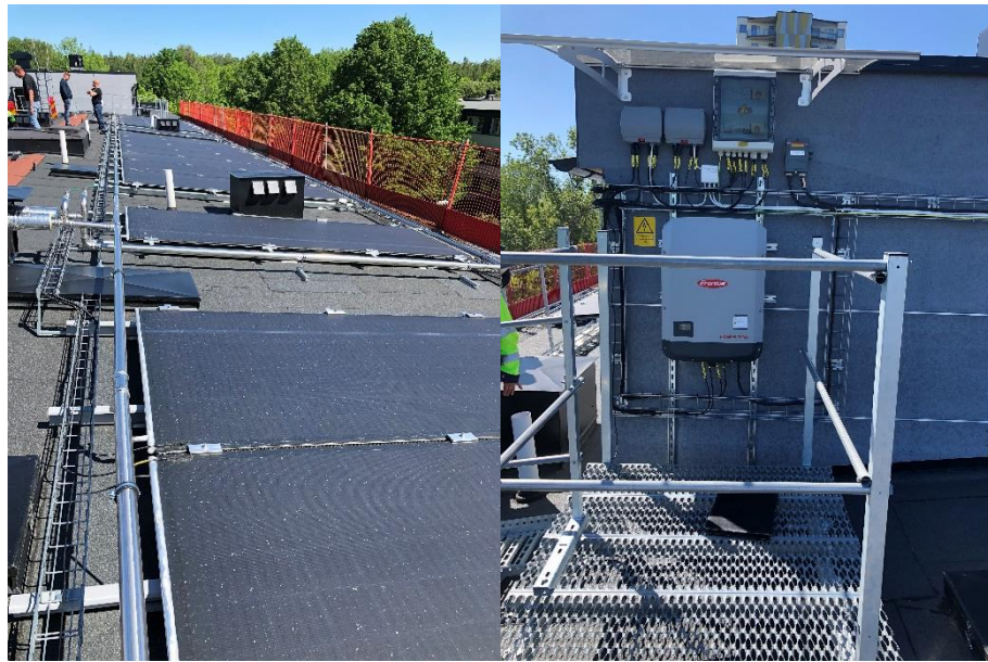
Figure 19: PVT system (RDP SE-PVT) installed on Alabastern (RDS SE1.1), left: PVT panels, right: PV inverter
