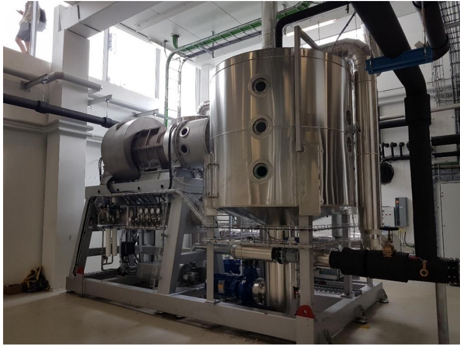
Figure 35: Water chiller installation of the 1 MW sea water-fed heat pump (RDP DK-WW1)
