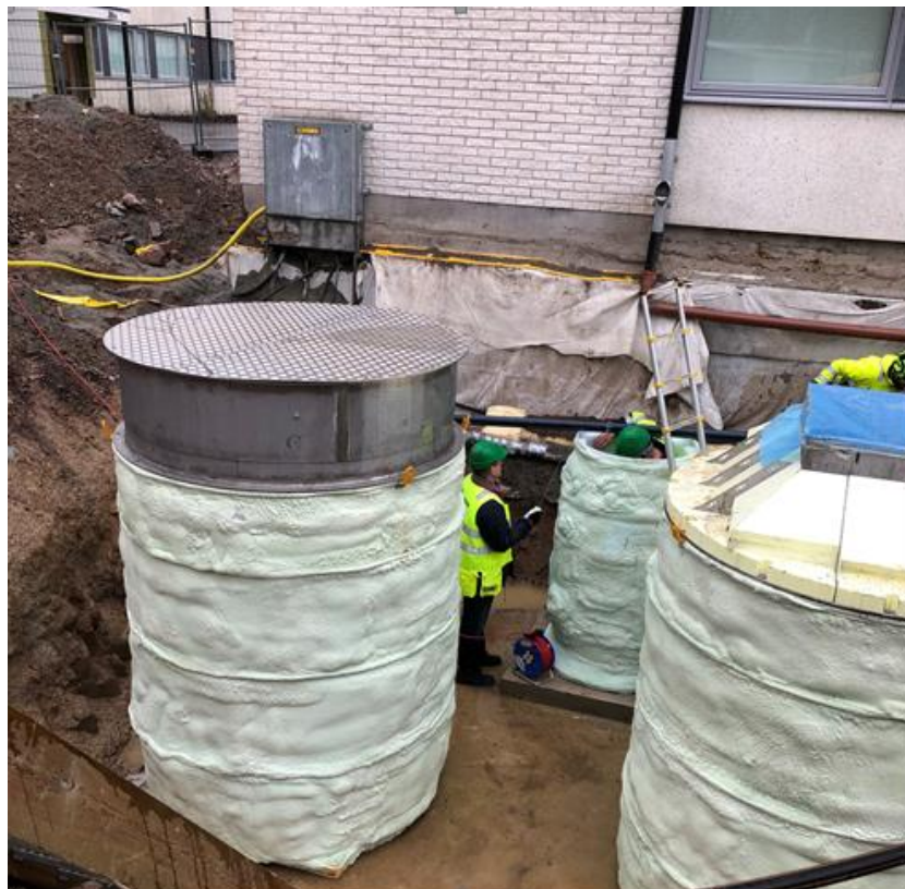
Figure 29: Innovative WW-HR facility (RDP DK-WW2) at RDS SE1.1. Heat exchanger module to the left, pumping unit in the middle and buffer tank with stirring device to the right. All done as prefab and pre-insulated manholes. 25
