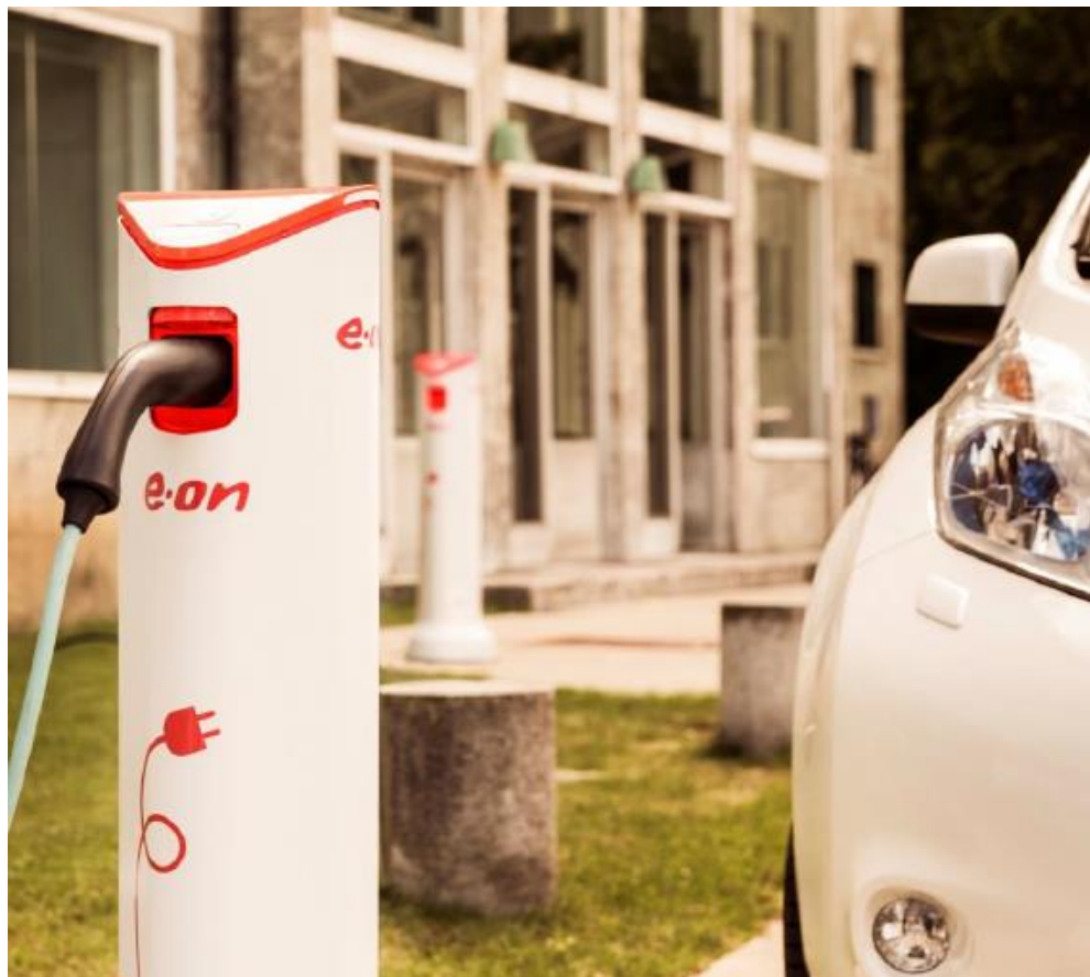
Figure 32: Example picture of charging pole of RDP DK-Ch in Aarhus 29
