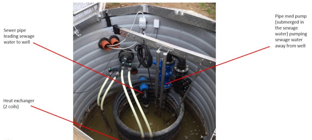
Figure 31: Prefab plastic manhole with integrated heat exchanger at RDS DK2 27
