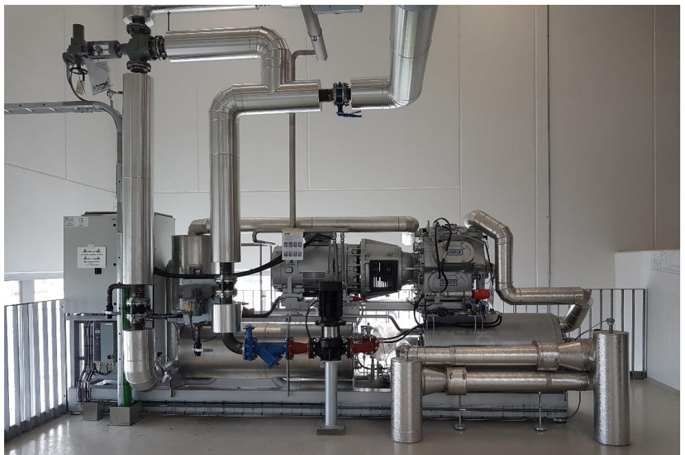
Figure 36: Ammonia chiller installation of the 1 MW sea water-fed heat pump (RDP DK-WW1)
