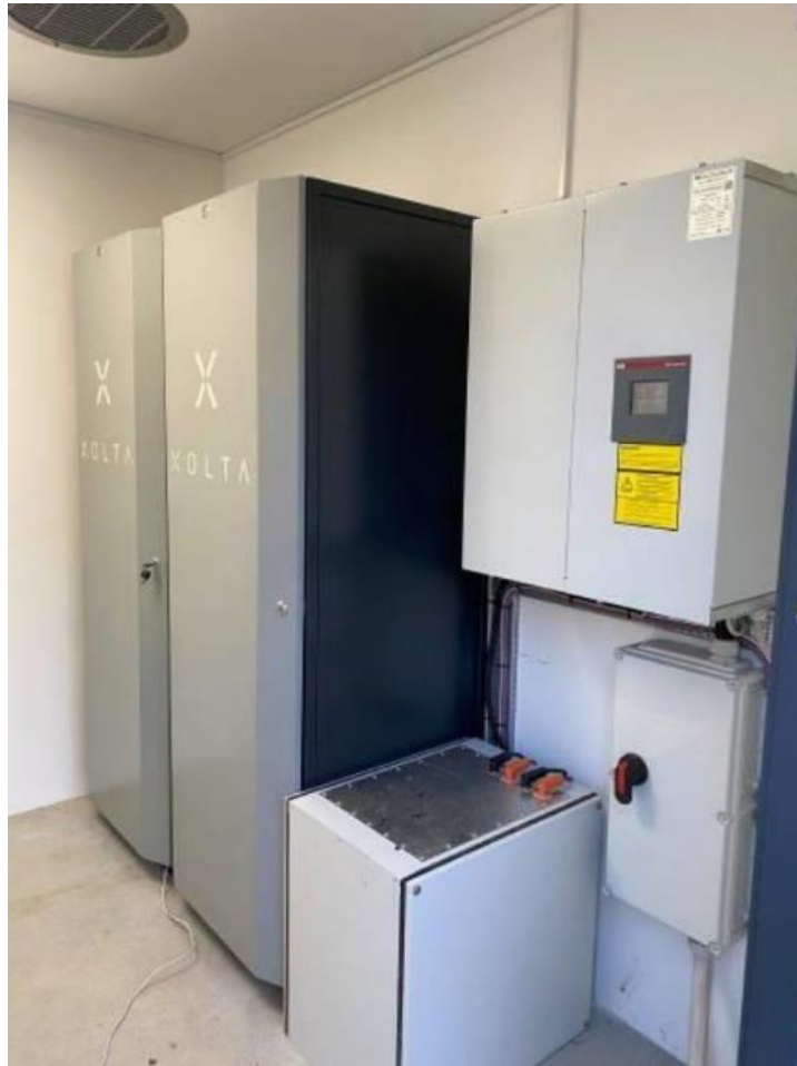
Figure 26: The two Battery storage racks, inverter and control system of the RDP DK-ST at RDS DK2 24 (left: new batteries with a capacity of 79 kWh; right: 2 nd life batteries from EV with a capacity of 35 kWh)
