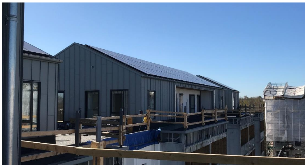
Figure 24: View of the installed PV system on the roof of a multi-apartment building in Rydevænget (RDS DK1)
